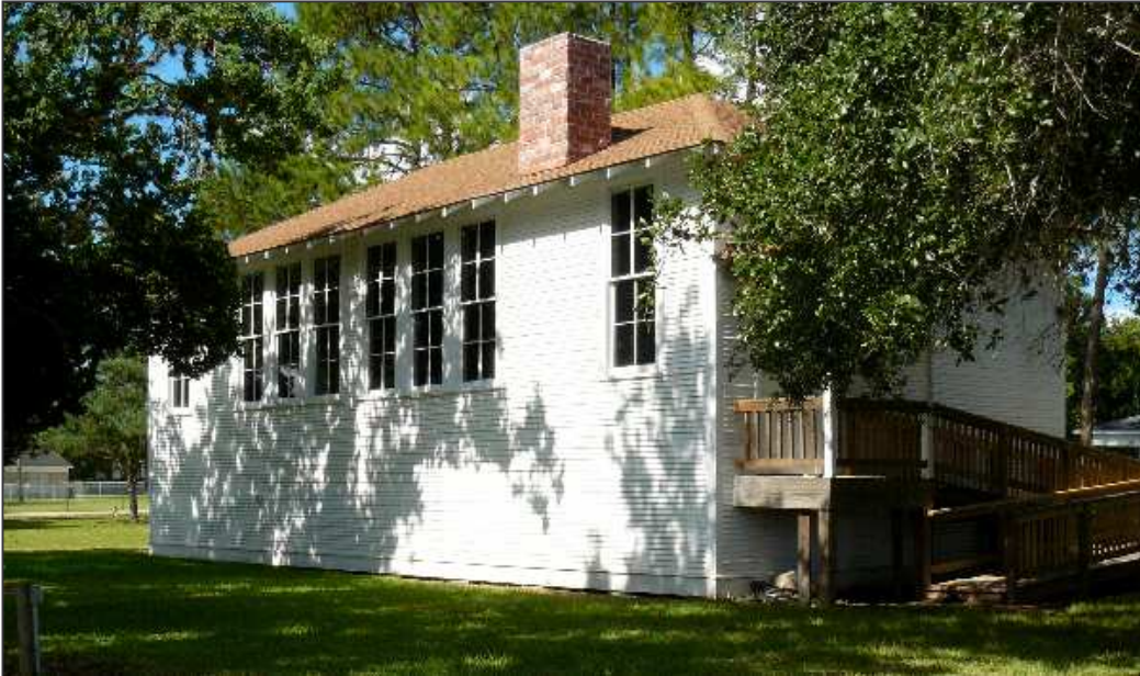
Exterior of the Columbia Rosenwald School during renovation, looking southwest, August 2009. Note the large windows on the east side of the building.
