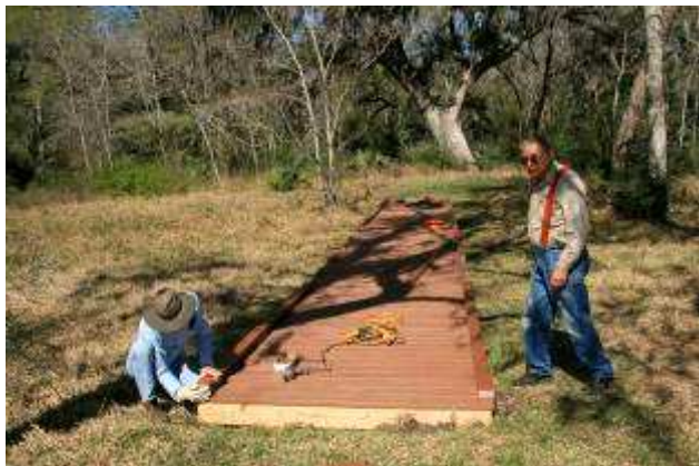
Archie Pratt and Kirby Rapstein putting finishing touches on a Bayou Loop Trail boardwalk.
