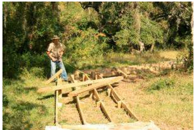
COT member and Crew Chief Kirby Rapstein working on a boardwalk section.
