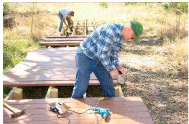
Don Van Dragt (in rear) and Gerald Forrest building a boardwalk on the Bayou Loop Trail.
