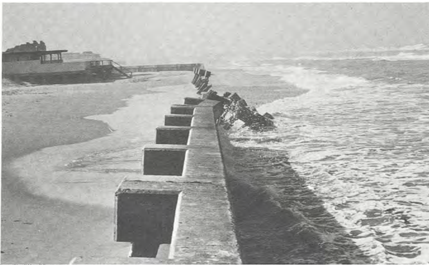
Figure 64. Seawall on south Padre Island, south of the National Seashore. Portions of the seawall have collapsed as a result of frequent attack by daily wave and tidal activity and as a result of less frequent but more intensive assault by very high tides accompanying tropical storms and hurricanes. Note the absence of a usable beach in front of the seawall.
