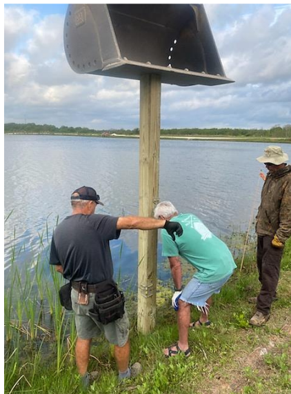
Left: Oron Atkins and George Valadez positioning support posts for one of the fishing piers. Below: Refuge staff with volunteers Tom Taroni and George Valadez admire their work.
